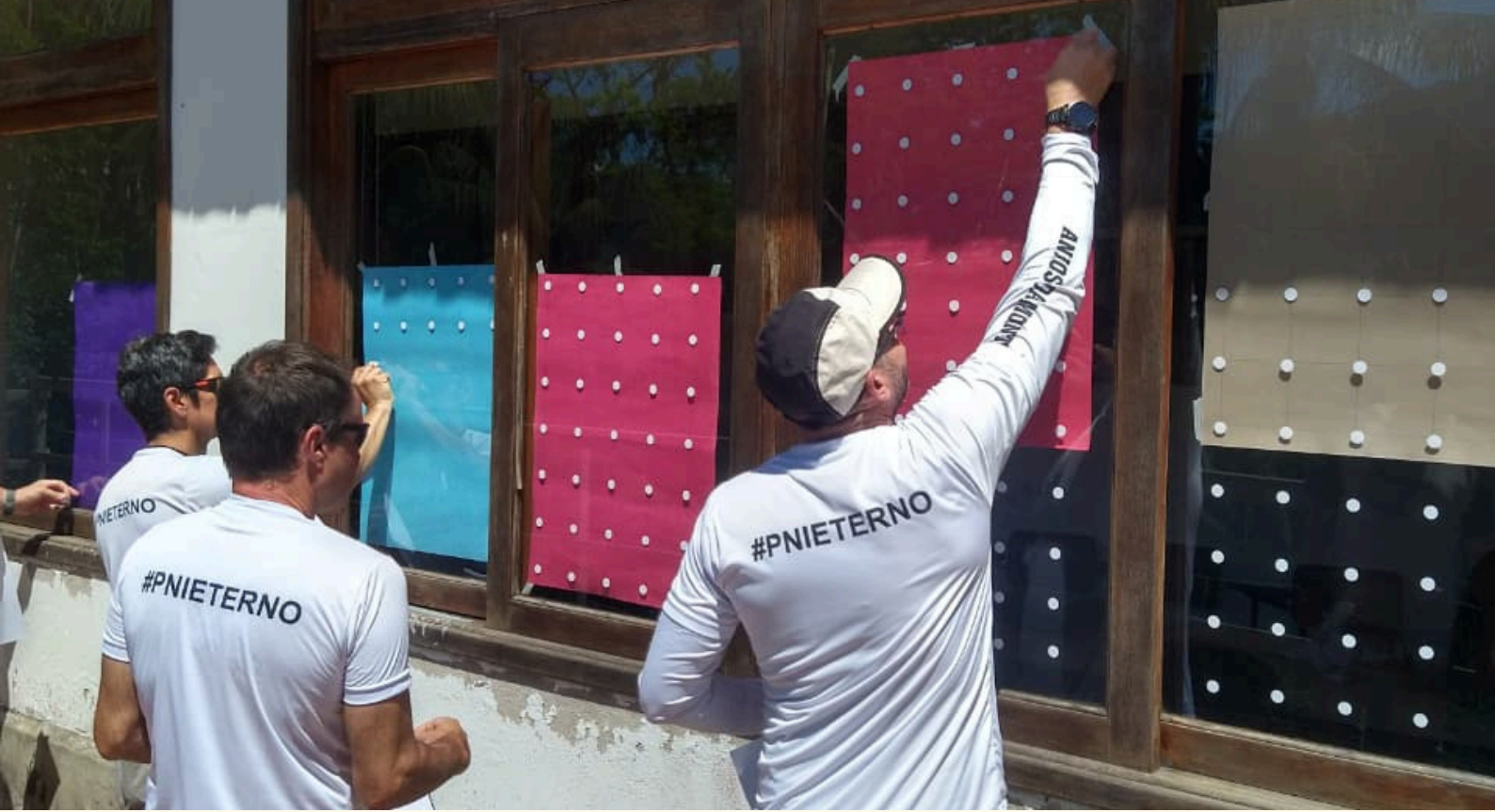
Employees of Itatiaia National Park participate in a collective effort to affix anti-collision stickers to the park's administrative headquarters windows.
